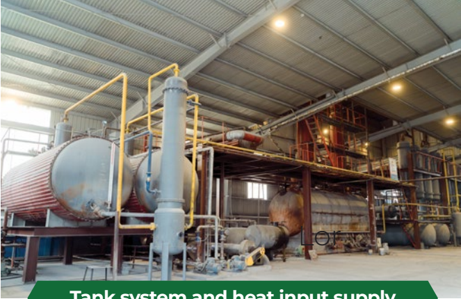
Tank system and heat input supply
